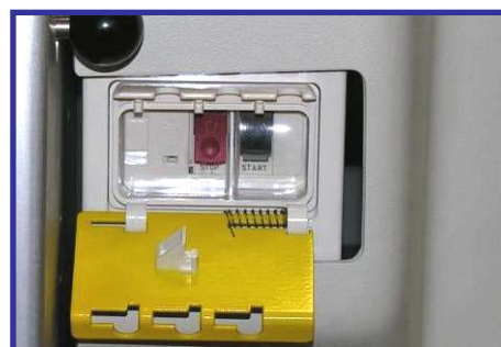
Interruptor de corriente principal
